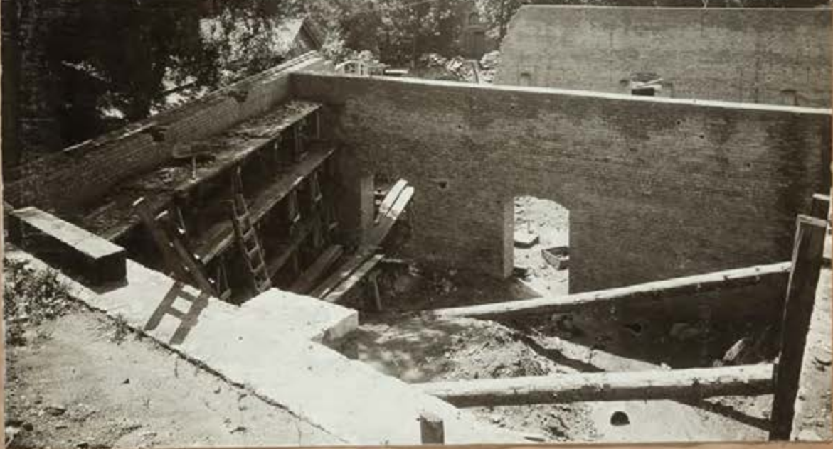
185. POWER HOUSE. MINNESOTA STATE CAPITAL CASS GILBERT, ARCHT. JULY 7, 1902. HAAS & WRIGHT, PHOTO.
